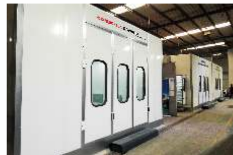
水性漆喷漆房 Water Based Paint Workshop
